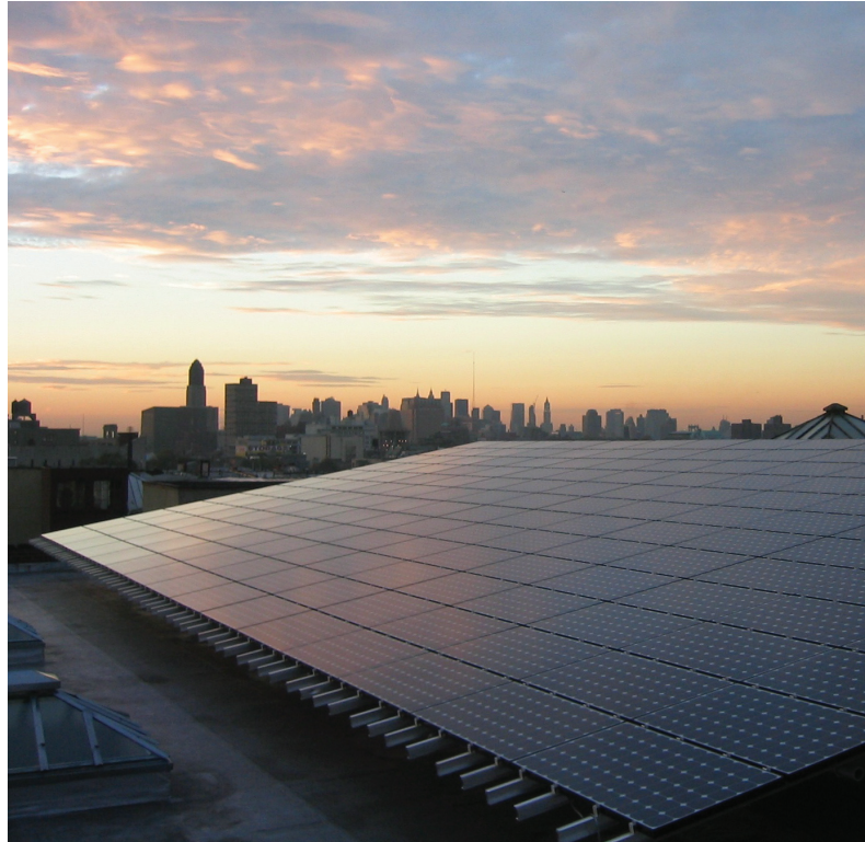
EF 14: Solar panels on the roof of Silvercup Studios in Brooklyn.
