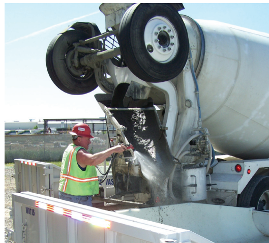
HT 13: Concrete washout water has a pH comparable to Drano® Clog Remover.
